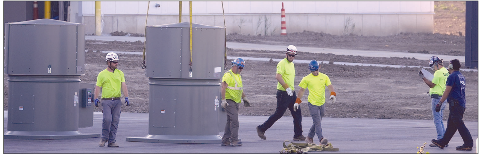
The GEM Mechanical Team set 86 exhaust fans plus two HVAC units on the roof of Ford Motor Co.'s under-construction electric vehicle facility in Northeast Ohio.
