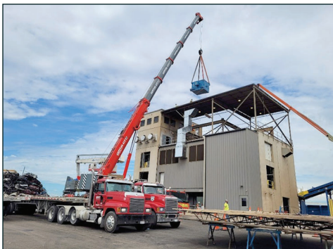
The upgrades at BlueScope Recycling will help it meet the demands of the second arc furnace at North Star BlueScope Steel.
