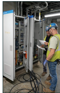
A complex HVAC system will control temperature and air flow for the motor and inverter.
