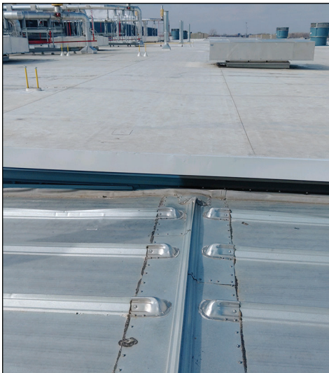
GEM HVAC technicians at present have to negotiate two roof systems – a standing seam roof and a rubber roof – as they service rooftop equipment at Ardagh.
