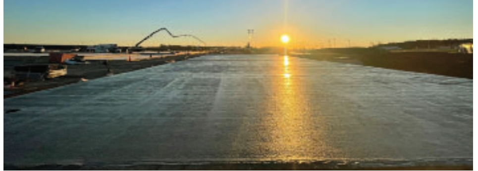
Limited lighting, trip hazards and changing light conditions are some of the issues that need to be addressed prior to an early morning pour.
